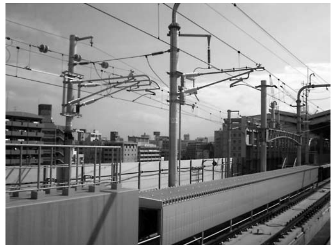
Kyushu Shinkansen new overhead contact wire equipment
