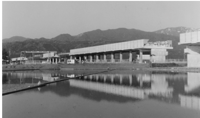
Construction of elevated section of Hokuriku Shinkansen in Toyama Prefecture due for completion in 2012 (Author)
