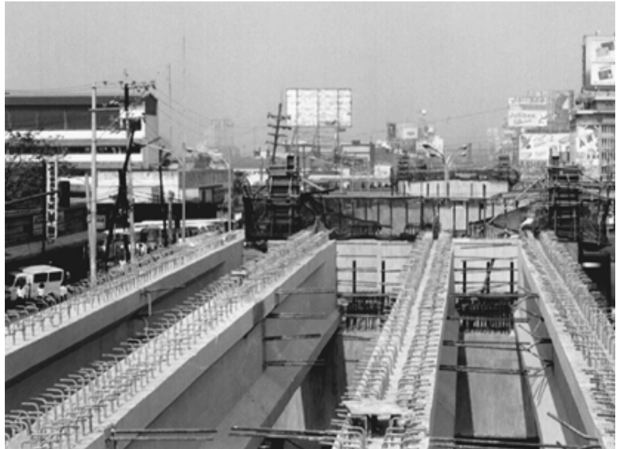
Newly-laid crossbeams just south of Cubao, Quezon City near intersection of LRT Line 2 and 3 (EDSA MRT Project)
